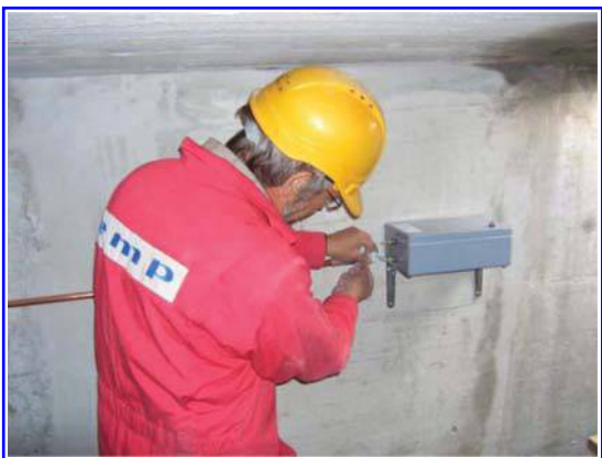
Figure 13a: Mounting of a LAS-meter measuring chamber at the inside wall of the bridge, field 2, and connecting it to the pressure tube, made of copper.
