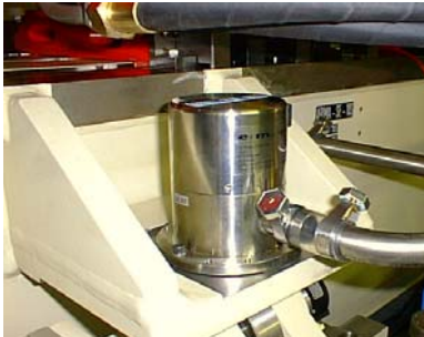
Fig. 1: HLS-Level sensor mounted on a girder.
